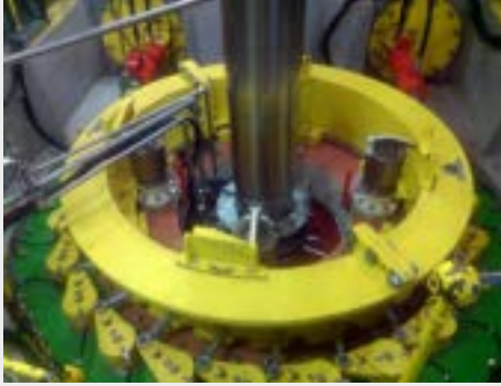
Figure 11: ENERGO-PRO Bulgaria EAD driving technical improvements in line with environmental standards – case study
